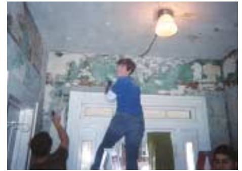
Making all things new. Sara Armstrong works to remove five layers of peeling wallpaper while on mission in Tennessee.
