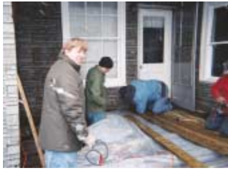
SPRING break? As snow flurries fall, Kevin Sheridan, John Nettles and Campus Minister Clark Carter install a new porch.
